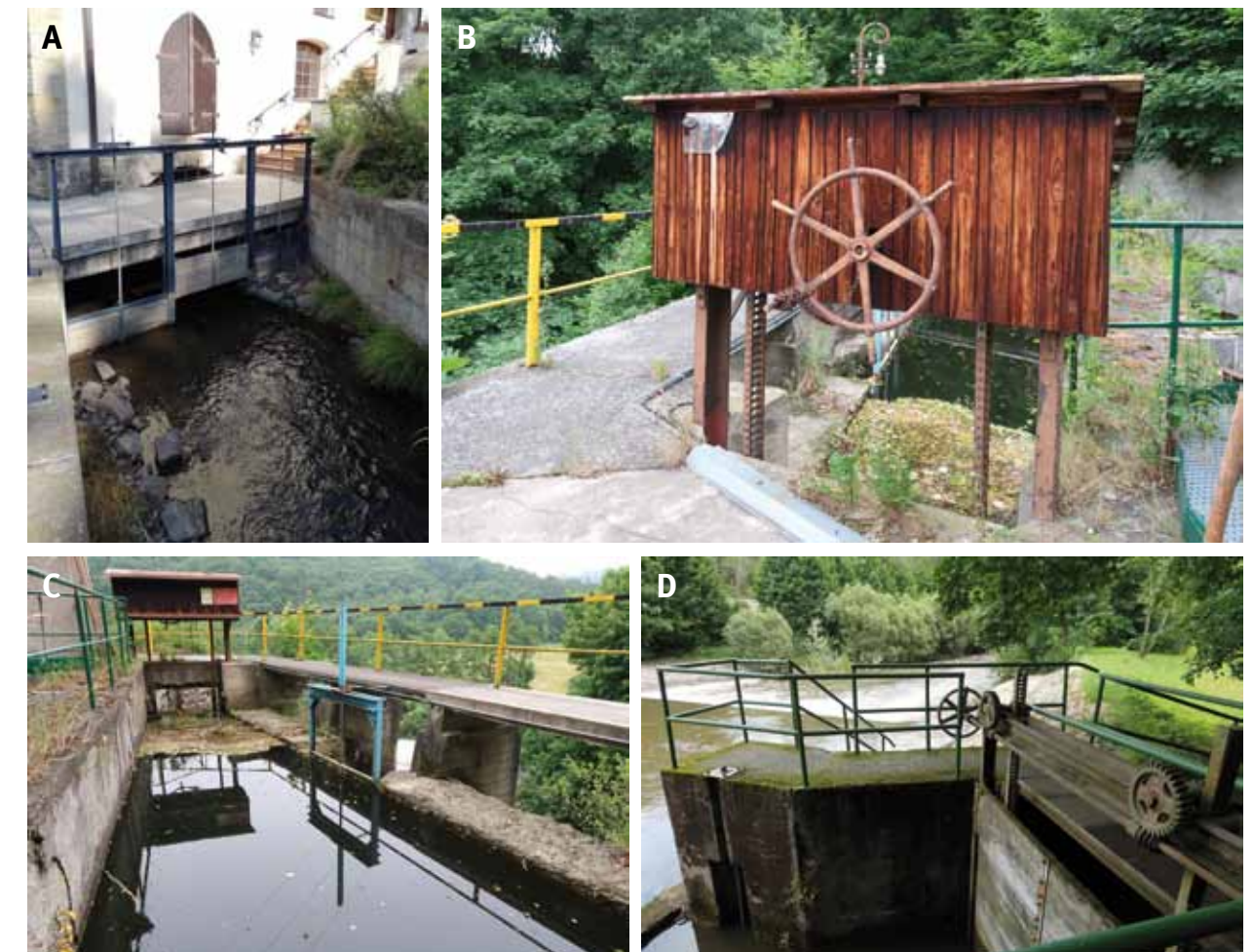
Fig. 4.94: Control structures details: (A) Chrudim, wood, hand-operated sluice gates; (B) the Weissshuhn Canal, an originally hand-operated sluice gate converted into electrically-powered; (C) the same place, right-bank residual outflow operated hydraulically; (D) mechanism for manual control of sluice gates from the side. Photograph by Radka Račoch, 2021.
