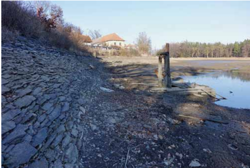
Fig 4.53: Zbýšov, stone riprap of the upstream dam side of Zbýšovský Pond. Photograph by Jindřich Frajer, 2018.
