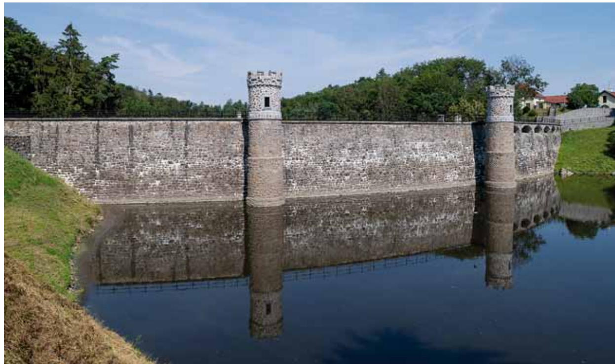
Fig. 4.9: The Pařížov dam (1909–1913) – control towers on the upstream side of the dam for the handling of inspection slide gate valves. Photograph by Viktor Mácha, 2020.
