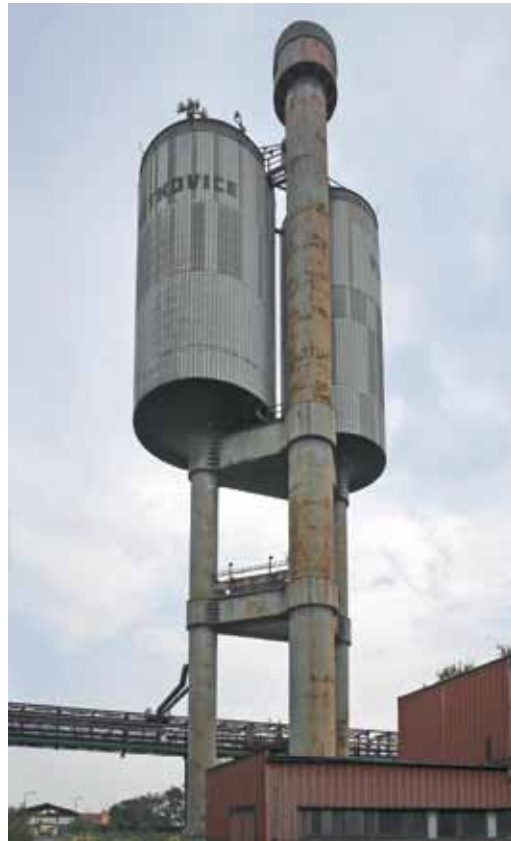
Fig. 4.222: Ostrava-Vitkovice – steel elevated water structure with two tanks. A steel elevated water tank typical for industrial companies, which, however, deviates from that era's production in terms of typology, structure and parameters. The structural design is different from the commonly built steel elevated water tanks from the production of the Vitkovice Ironworks (water tanks in Ostrava-Hladnovo). What is unique is each tank being carried by a separate shank and a lift shaft situated in the third separate shank, which has been documented in the Czech Republic only in three cases. At the same time, it is one of the elevated water tanks with the largest volume in the Czech Republic. In the third national competition for the best construction with supporting steel structure organised by the Czech Association of Scientific and Technical Societies it won the main prize in the category of Technological structure for 1983. The water tank is also a dominant landmark and an important orientation point. The project and pre-production preparation was provided by Hutní projekt Praha, Ostrava plant (the general designer was Ing. Antonín Kozák) and VŽKG, k. p., Ostrava, Ing. (the vessels were designed by Pavel Klimeš) (Devátý, 1983, Soušek, 1982). Photograph by Michaela Ryšková, 2016.
