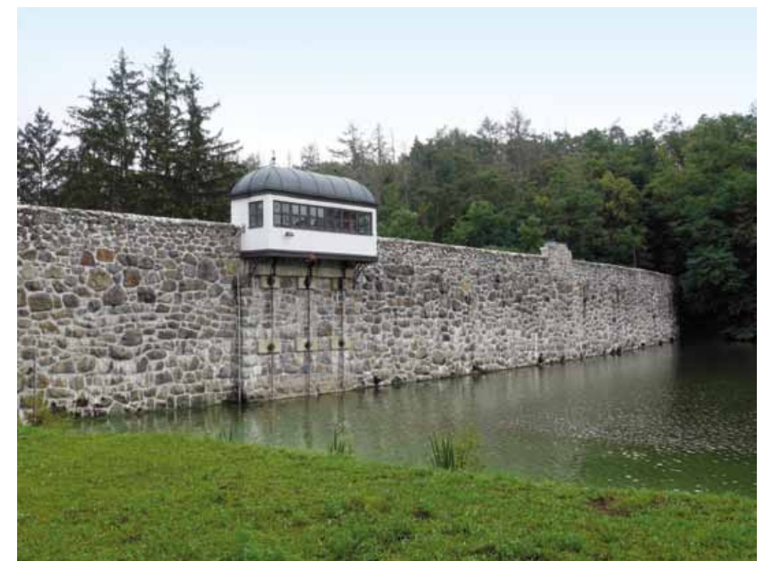
Fig. 3.7: The Jevišovice dam (1884–1896) is one of the two oldest masonry-built dams in the Czech Republic. The authenticity of form has been disrupted by modifications to the crest of the dam and the addition of an engine room containing the control mechanisms for the bottom outlets. Historical postcard, collection of Michaela Ryšková. Photograph by Michaela Ryšková, 2020.
