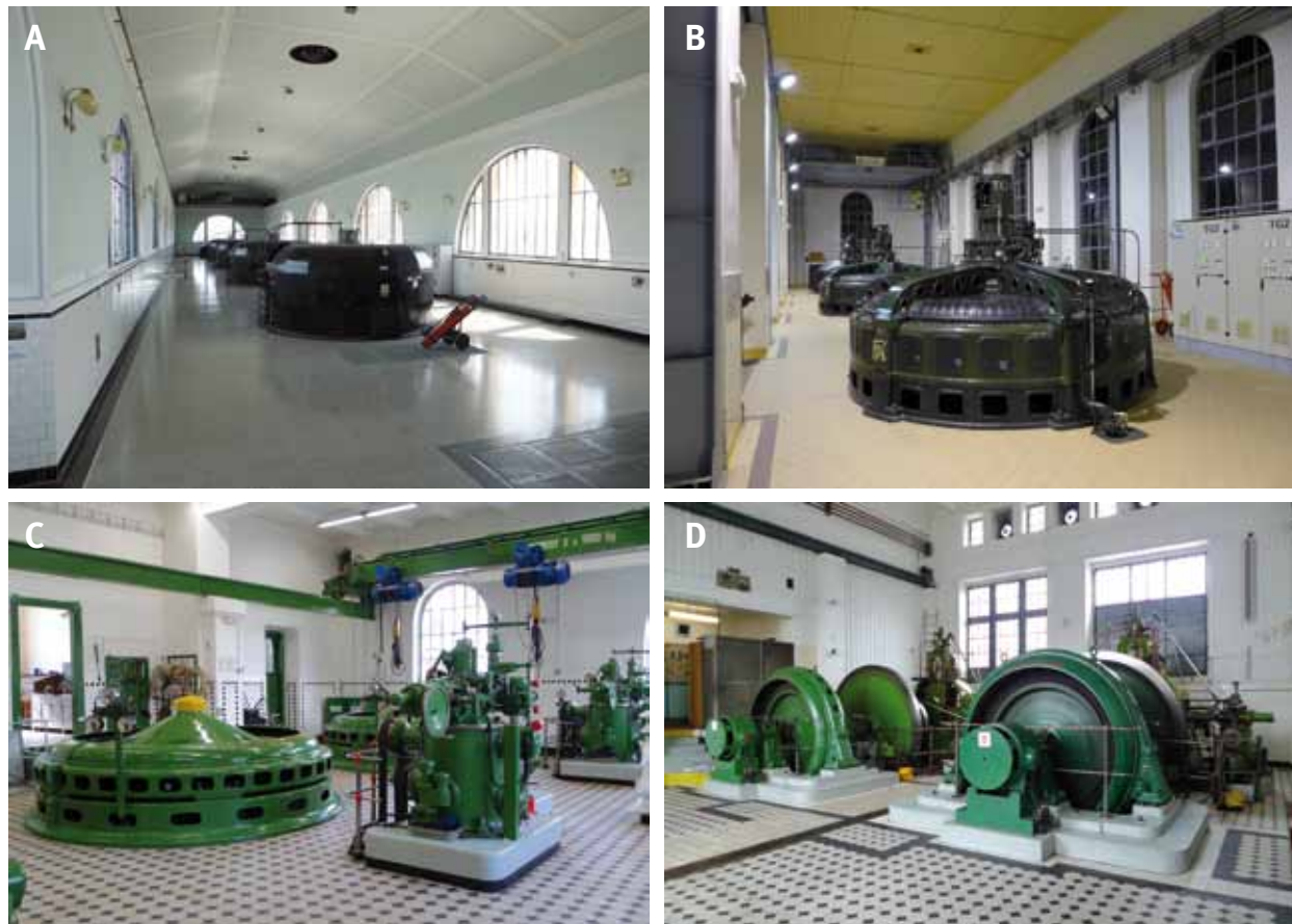
Fig. 4.159: Machine rooms: (A) Miřejovice SHPP; (B) Kroměříž SHPP; (C) Hradec Králové – Hučák SHPP; (D) Hradec Králové SHPP. Photograph (A) by Brno University of Technology, Faculty of Civil Engineering, 2014; (B) by Miloš Matěj, 2014; (C) and (D) by Michaela Ryšková, 2010.
