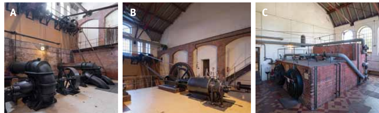
Fig. 4.269: Prague-Bubeneč. Old wastewater treatment plant: (A) and (B) steam engine machine room; (C) boiler room. Photograph by Viktor Mácha, 2019.
