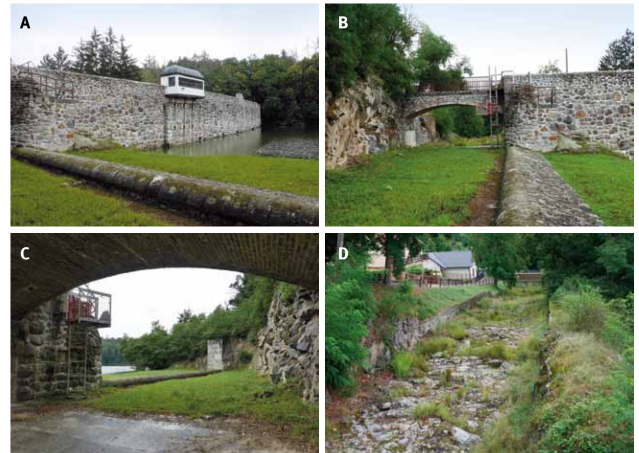
Fig. 4.28: The Jevišovice dam (1884–1896) – masonry gravity dam. Top left, overflow edge of an uncontrolled side safety spillway. Top right, overflow edge and drop structure. Bottom left, view into the drop structure from under the bridge. Bottom right, the chute. Photograph by Michaela Ryšková, 2020.
