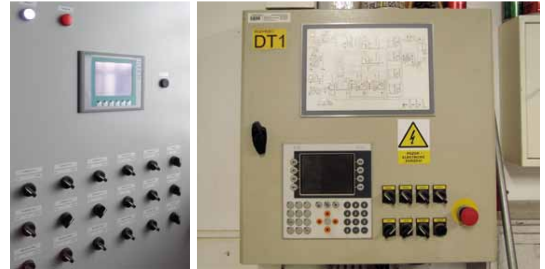
Fig. 5.29: Now historical equipment for the management of the operation of the water treatment plant. Photograph by Miloš Rozkošný, 2021.
