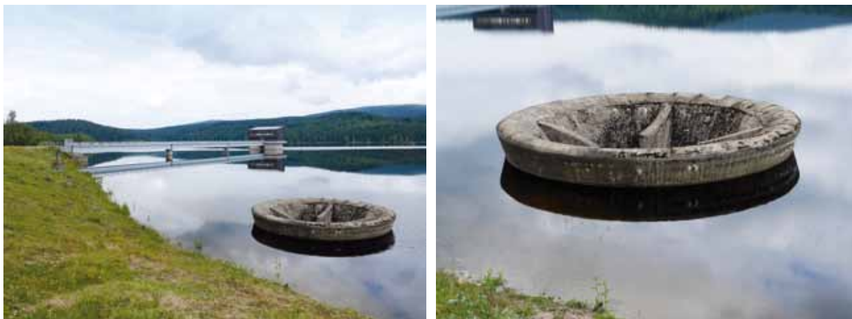
Fig. 4.30: The Josefovo Důl dam (1976–1982) – earthfill dam, shaft safety spillway. Photograph by Michaela Ryšková, 2020.
