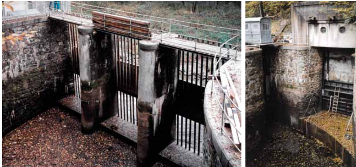
Fig. 4.143: Spálov derivation SHPP – inlet structure, state without water at the time of repair in 1998. Photograph by Brno University of Technology, Faculty of Civil Engineering, 1998.
