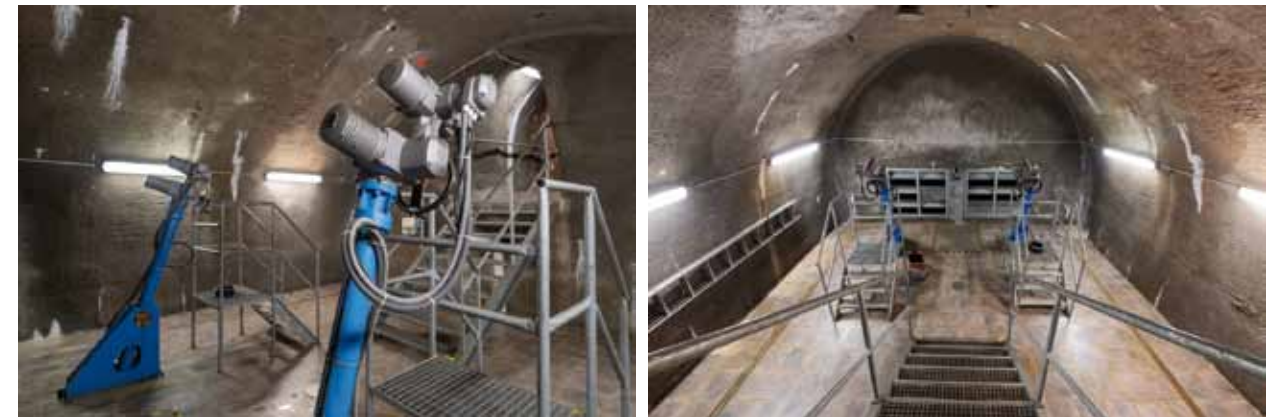
Fig. 4.10: The Pařížov dam (1909–1913) – handling of operational radial gates of bottom outlets (DN1200) located in the by-pass tunnel. Photograph by Viktor Mácha, 2020.
