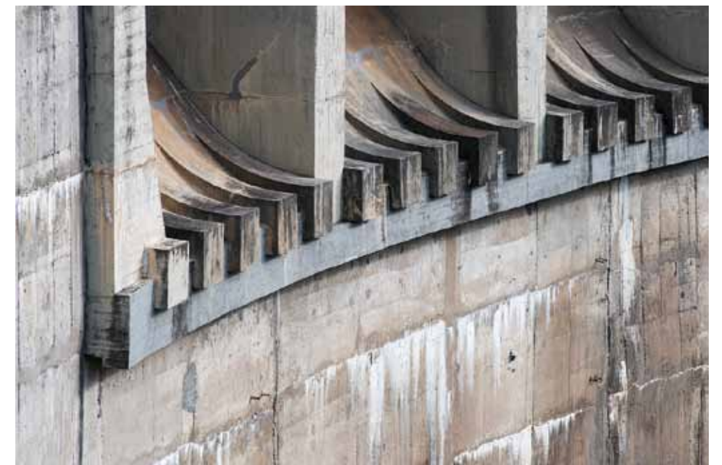
Fig. 3.16: The Vrchlice dam (1966–1970), punctuated by the control blocks at the dam crest, contrasting with the monumental outward-facing surface of the dam. Photograph by Viktor Mácha, 2020.
