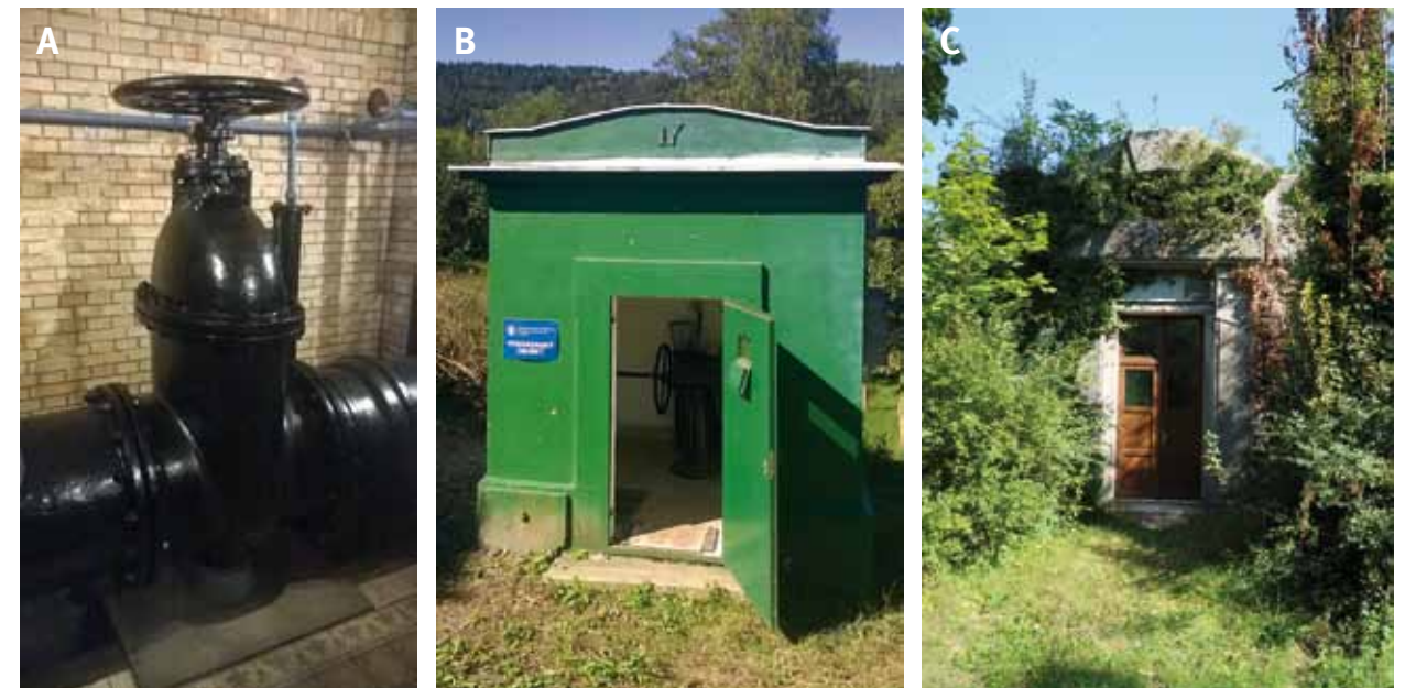
Fig. 3.3: Březová aqueduct no. 1: (A) aqueduct supply valve; (B) gate valve chamber; (C) entrance to the Holé hory 2 water tank; cast iron long-distance aqueduct for drinking water (57 km), preserved in its original form with the exception of the addition of a remote control system to operate the machinery. Photograph (A, B) by Miriam Dzuráková, 2018 and (C) by David Honek, 2019.
