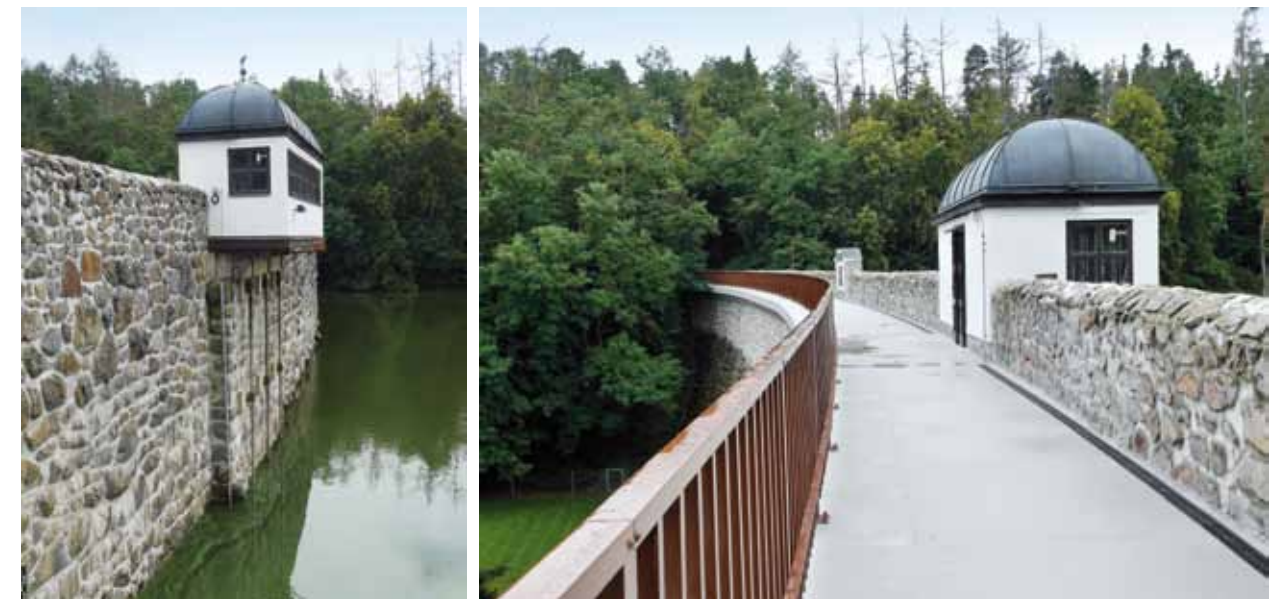
Fig. 5.25: The Jevišovice dam – structure for handling bottom outlets. Photograph by Michaela Ryšková, 2020.
