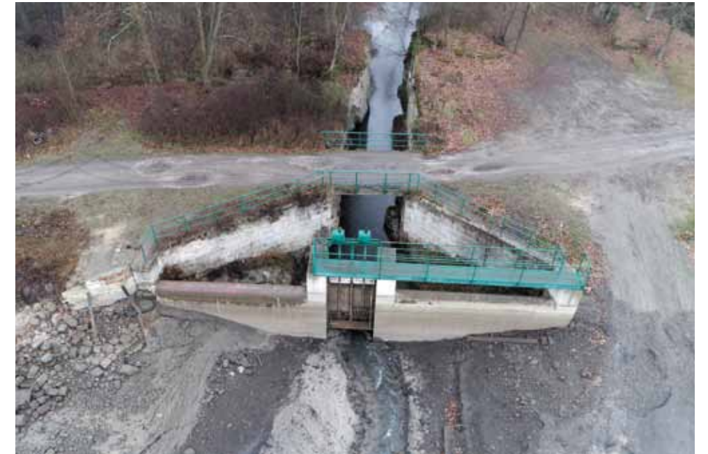
Fig. 4.56: Holany, Holanský Pond – the main outlet with a discharge to the sandstone rock gully. Photograph by J. Vidman, 2018.
