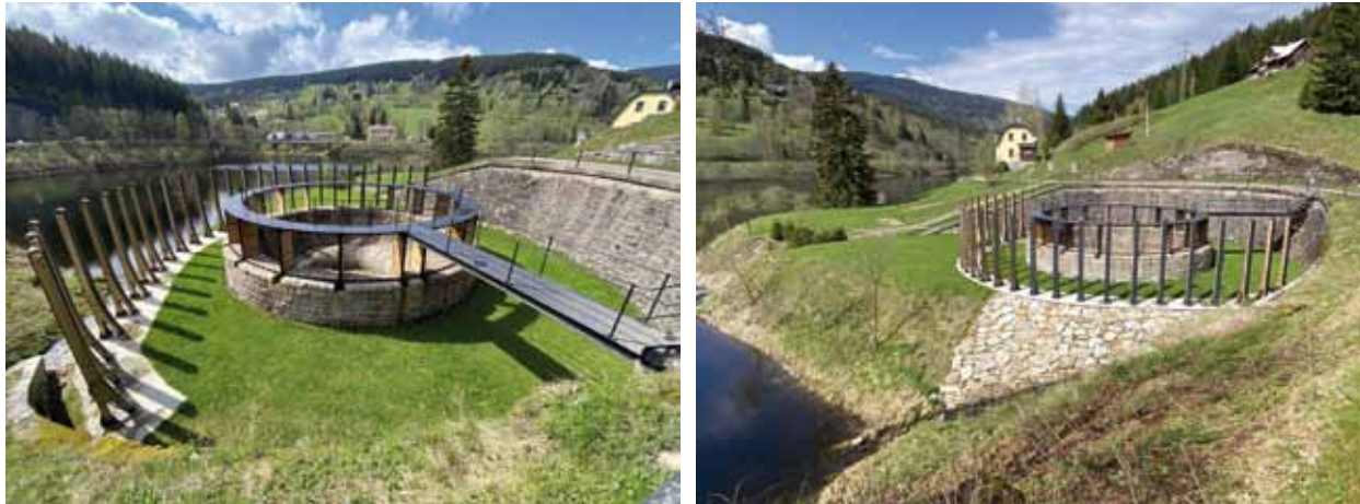
Fig. 4.29: The Labská dam (1910–1916) – masonry gravity dam, shaft safety spillway which was being reconstructed in 2017–2019. Photograph by Radka Račoch, 2021.
