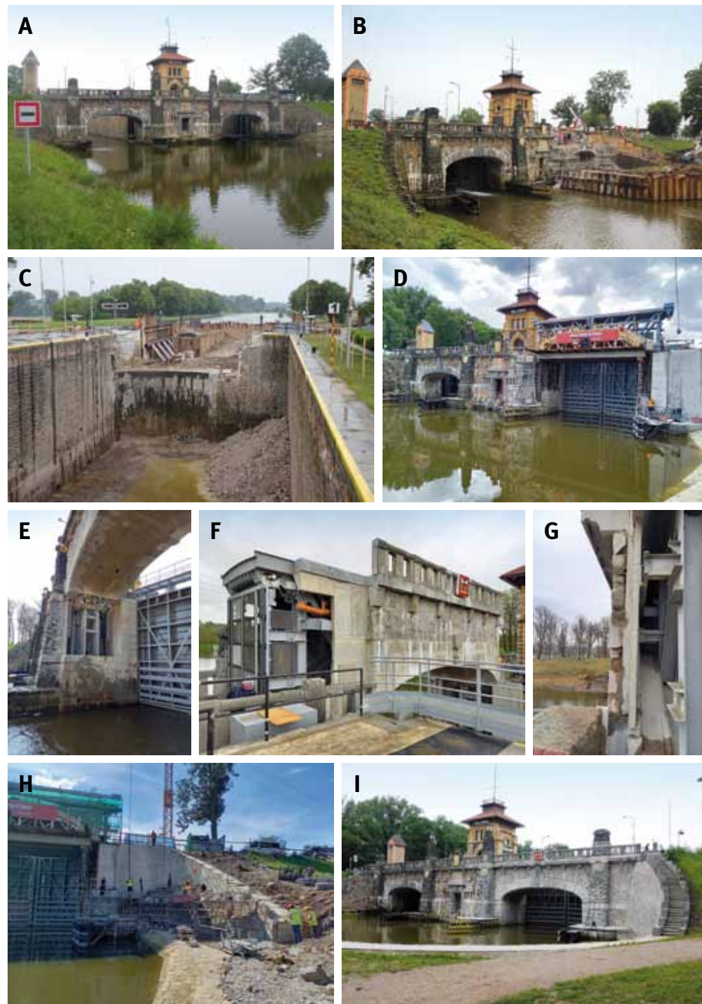
Fig. 5.4: Hořín – lock in the course of reconstruction: (A) state before the reconstruction; (B) and (C) dismantling of original structures and stone cladding; (D) to (F) new moveable bridge and lock chamber structures; (G) and (H) installation of the original facing on a new reinforced concrete structure; (I) current lock appearance. Photograph (A) – (H) by Otakar Hrdlička, 2021; (I) by Michaela Ryšková, 2021.
