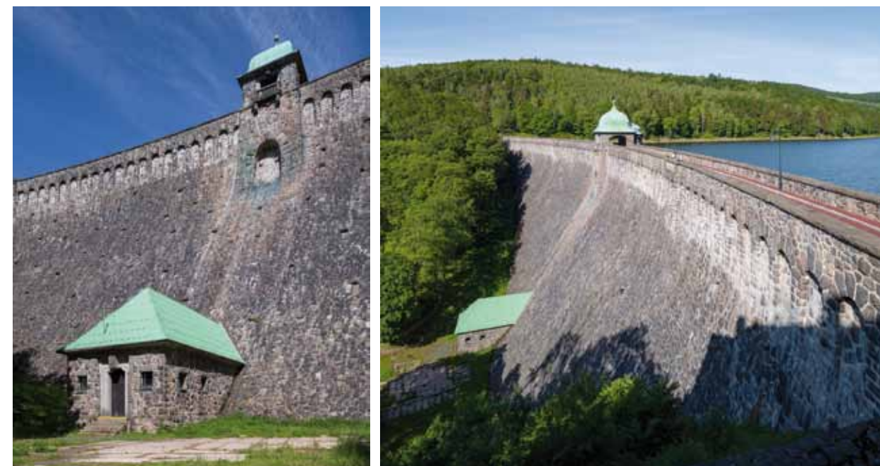
Fig. 4.8: The Janov dam (1911–1914) – an example of a masonry dam. Photograph by Viktor Mácha, 2020.
