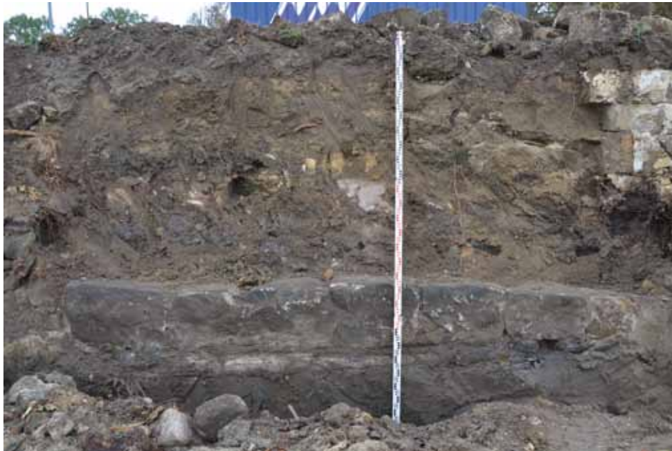
Fig. 4.54: Holany, Holanský Pond – construction of the dam with the revetment of the upstream face, the sandstone masonry is founded on the beam grid from the beginning of the 16th century. Photograph by Miroslav Kolka, 2018.
