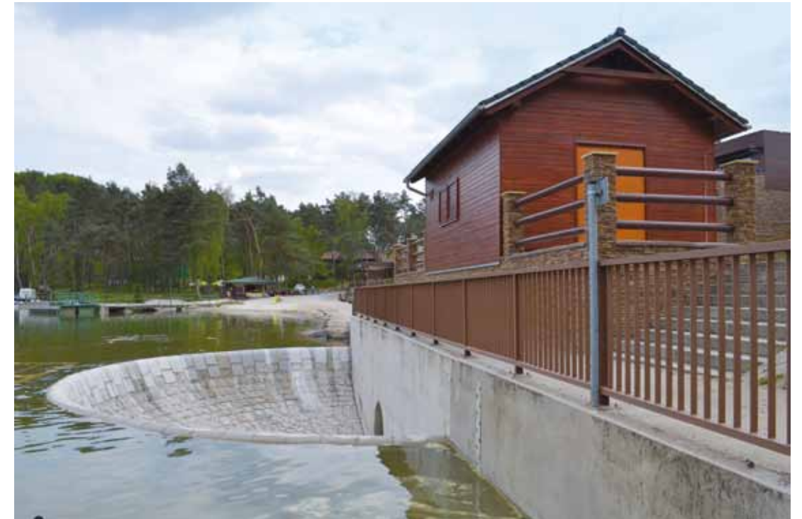
Fig.4.31: Mácha Lake (1366) – straight earthfill dam from local materials, detail of fountain safety spillway. Photograph by Miroslav Kalka, 2016.
