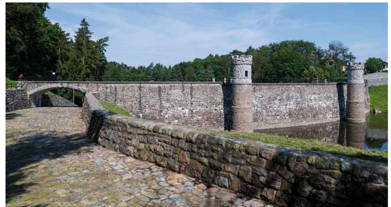
Fig. 4.11: The Pařížov dam (1909–1913) – overflow edge of the side safety spillway and drop structure which behind the bridge follows the cascade. Photograph by Viktor Mácha, 2020.
