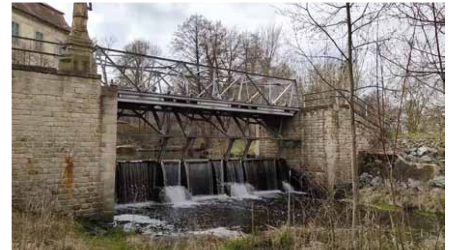
Fig. 4.107: Křimice, a shutter weir with overhead bridge on the Mže River. Photograph from the Brno University of Technology archive, 2018.
