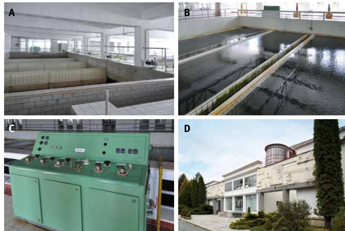
Fig. 4.232: Vítkov-Podhradí – water treatment plant: (A) filtration hall; (B) filtration tanks; (C) original control panel. Photograph by David Honek, 2019; (D) relief (for more photographs see Chapter 3.2, art-historical value). Photograph by Roman Poláček, 2019.
