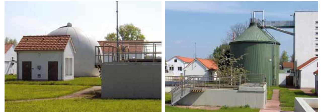
Fig. 4.256: Sludge handling and disposal within a WWTP – sludge-digestion tanks and biogas collection. Photograph from the TGM WRI archive.
