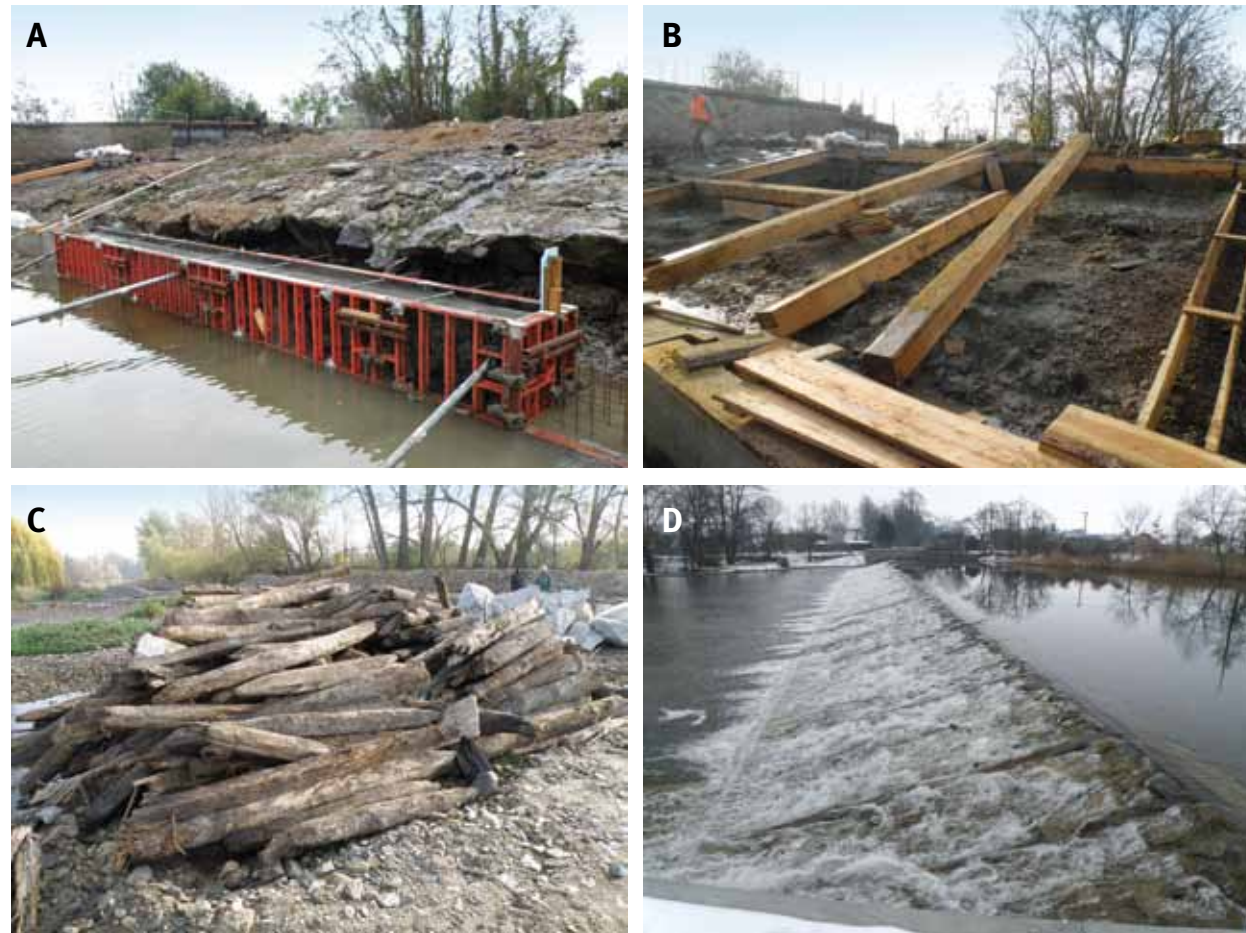
Fig. 5.5: Znojmo-Oblekovice – reconstruction of the weir in Oblekovice on the Dyje River: (A) foundation of a new weir heel, October 2018; (B) replacement of the weir body beam grid, November 2018; (C) original parts of the wooden beam structure; (D) reconstruction completed, January 2019. Photograph by Miriam Dzuráková, 2018, 2019.
