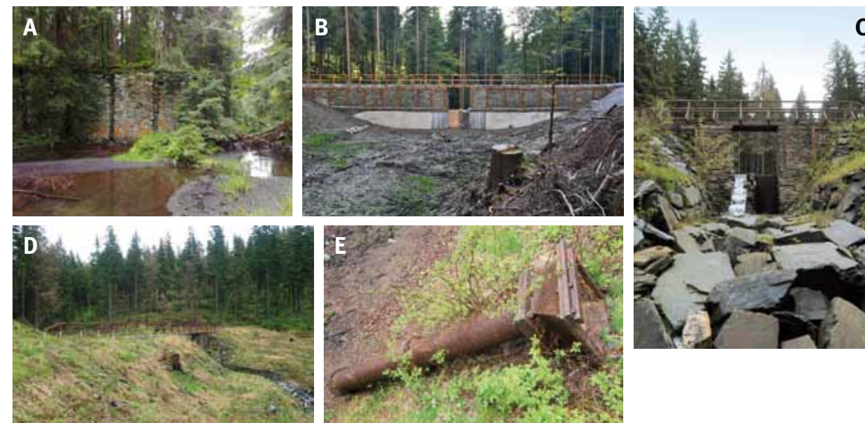
Fig. 5.11: Žďárský Potok, renewal of the splash dam on Splavský Brook: (A) remnants of the original dam; (B) repaired dam from the upstream side; (C) middle part of the dam with the flow section; (D) overall view of the dam from the downstream side; (E) original outlet piping. Photograph (A) and (B) taken from: Rymarousko, 2021; (C), (D) and (E) by Martin Caletka, 2021.
