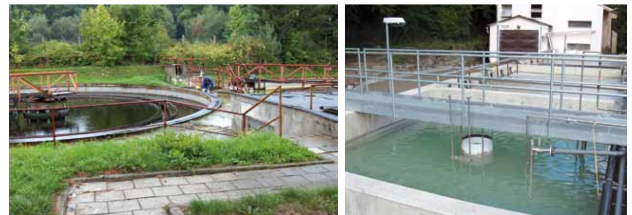
Fig. 4.253: Settling tank. Photograph from the TGM WRI archive.
