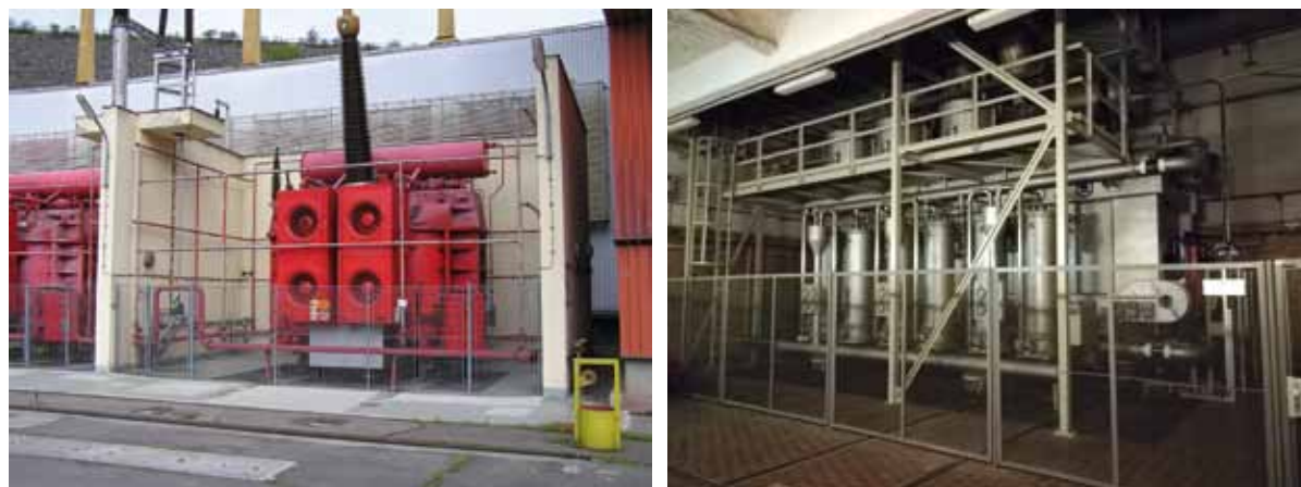
Fig. 4.180: Block transformers: (A) Dalešice PSHPP; (B) Dlouhé Stráně PSHPP. Photograph by Brno University of Technology, Faculty of Civil Engineering, 2019.
