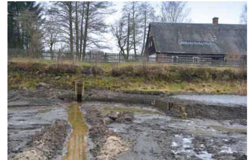
Fig. 4.64: Markvartice near Jablonné v Podještědí, Markvartický Pond – the bottom outlet of the idle discharge with a monk outlet, upstream face with typical revetment from sandstone blocks; state after the pond drawdown. Photograph by Miroslav Kolka, 2014.
