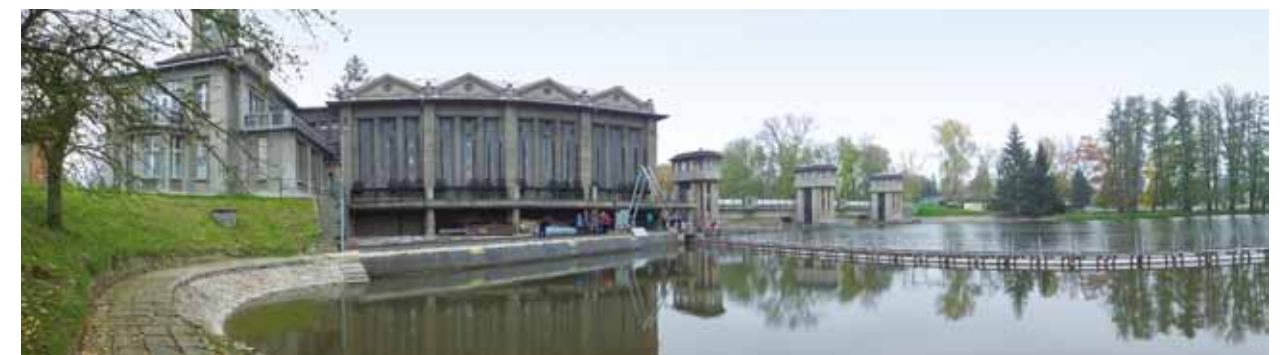
Fig. 4.129: Poděbrady SHPP – an inlet structure. Photograph by Brno University of Technology, Faculty of Civil Engineering, 2014.
