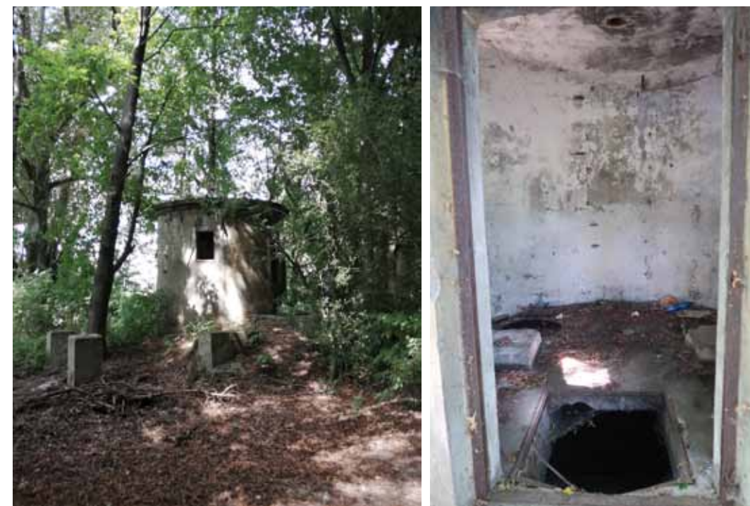
Fig. 5.27: Selmice (near the premises of the stud farm in Kladruby nad Labem) – the rest of the structures of the historical pumping station of irrigation water. Photograph by David Honek, 2021.
