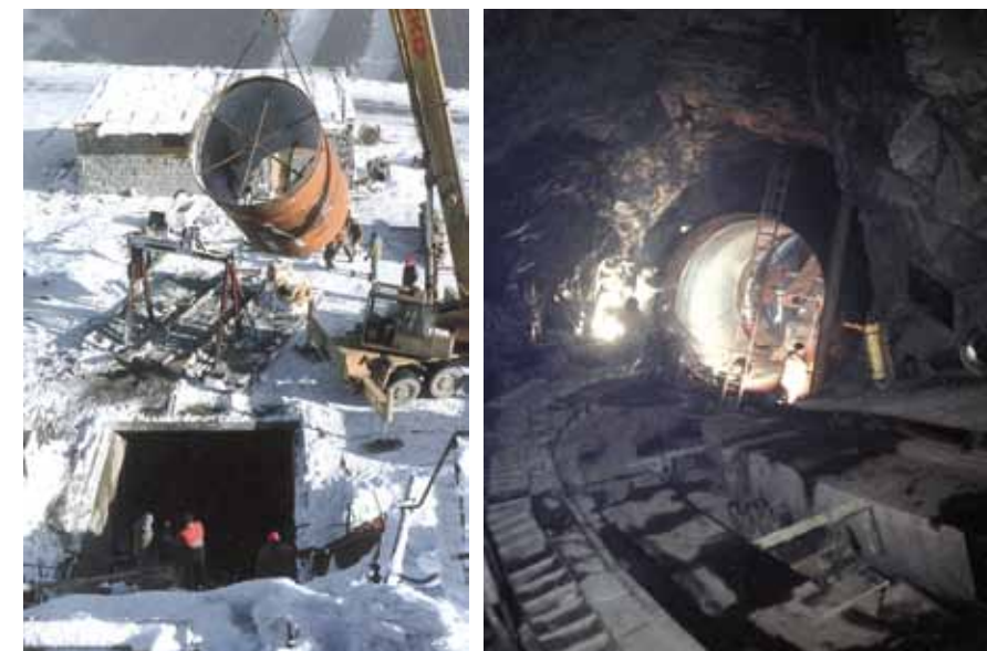
Fig. 4.151: Dlouhé Stráně PSHPP – positioning of steel armour into the inlet gallery of turbines (taken from: Höll, 1997).
