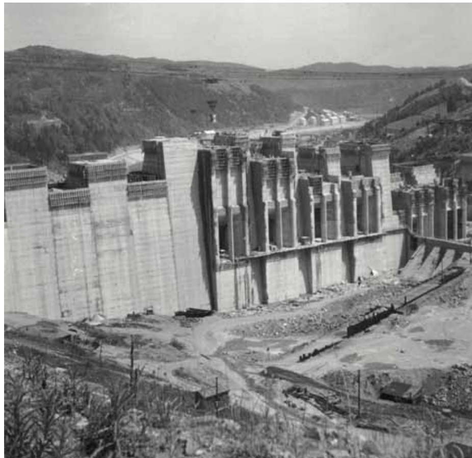
Fig. 4.144: Orlík HS – under construction, detail of blocks with inlets to the HPP. Photograph by Brno University of Technology, Faculty of Civil Engineering.
