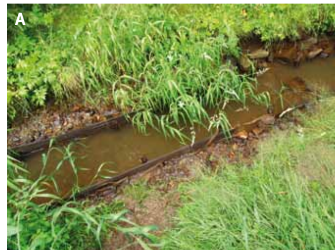
Fig. 5.12: Blatná Water Ditch – damaged sections of the water ditch: (A) affected by erosion and washing out; (B) endangered and damaged by woody plants in the proximity of the race trough. Photograph by Miloš Rozkošný, 2020.
